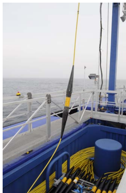
Figure 2: The two photos, a) and b) show installation and equipment in connection with the backbone cables and the two photos, c) and d) show installation equipment for the seismic cables.
