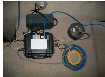
Figure 5 - View of the acelerographic station ACL2, located in the drainage gallery of block BG1 (elevation -28 m), showing the digitizer (left foreground), the uninterruptible power supply (behind of the digitizer), the switch (above of the digitizer) and the accelerometer (on the right).
