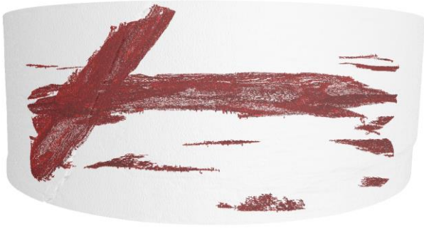
Figure 2. Transparent 3D view of the L300 CT result. Cracks are segmented (red colour).
