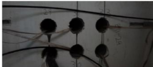
Figure 2 Photo of six PVC conduits like the ones used to host the fibre-optic cable used by our experiment. The photo was taken in a service manhole and shows how the telecommunication cables are laying at the bottom of the PVC conduit, which is surrounded by concrete.
