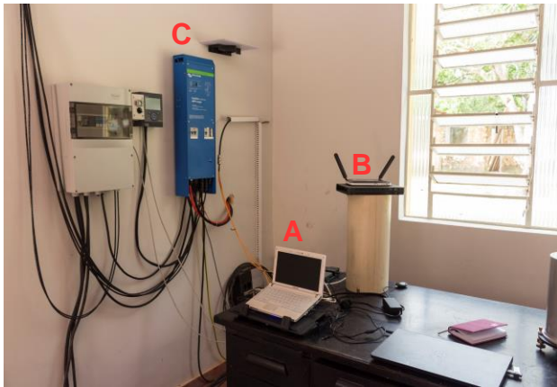
Figure 3 – New laptop (A), 3G router for internet (B) and energy management equipment (C) in TTB office.
