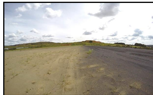
Figure 1: Contact between the flotation tailings and magnetite sand used to make heightening of BR dam.
