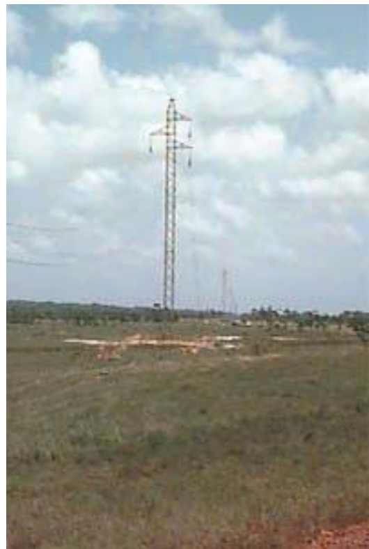
Fig.4: A TL of 69kV (Tartarugalzinho – Calçoene/ Eletronorte) with 126km of long using guard cable OPGW 14.5mm
