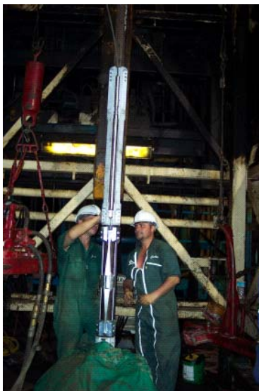
Figure 2 - Full deployment of the microseismic sonde before anchoring on the tubing. The tool, characterized by a mono-conductor telemetry, fits in the treatment well, with an identical installation as for permanent pressure gauge. The sensors assembly includes three orthogonal 28Hz geophones mounted on a bow spring blade.
