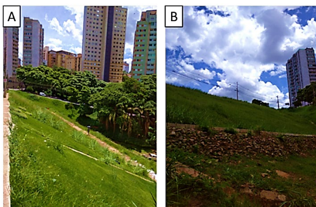
Figure 2 - Contextualization of the structure. A: Field photo of the crest region, oriented from the right abutment towards the left abutment. B: Field photo of the downstream region, oriented toward the crest and left abutment of the structure.
