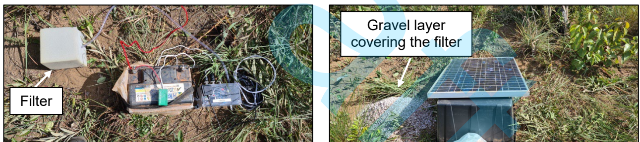
Figure 5 – Typical installation of one of the temporary elements: Left – RS&Boom connected to the battery and filter; Right – Protective box for the equipment, a layer of gravel covering the filter, and a solar panel.
