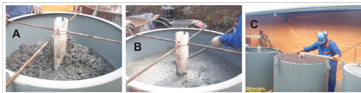
Figure 7 – Construction of well logging tower blocks. (A) Filling with controlled density blend; (B) Homogenization of filling material; (C) Finishing.
