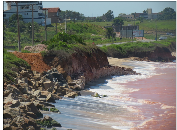
Figure 9 – Photograph showing road maintenance due to the present-day marine bluff erosion process taking place on Maimbá beach (March, 2015). The sea water color indicates the presence of fine sediment eroded from bluffs. Photograph source: Labogeo - 06/06/2016.
